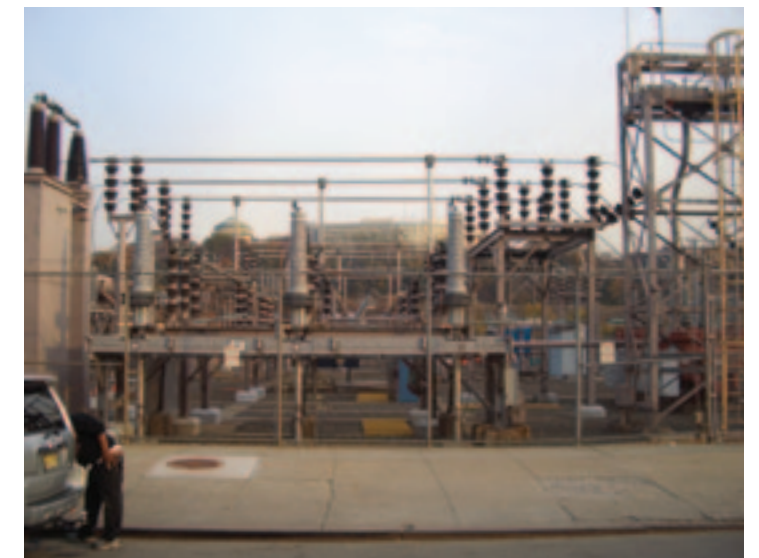
Fig. 11: Power distribution facility between West 201 st and West 202 nd Streets
